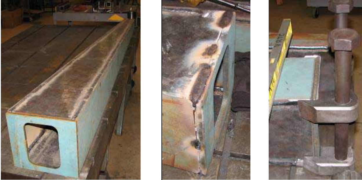
Figure 4.3: Left: Base Plate is added to the end. Middle: Base plate is welded to the Outboard Beam in the locations that the Hinge Brackets will overlap. Right: Hinge Brackets are being jugged up to weld. The bolts shown in the photo were removed and a aluminum jig was inserted into the holes to assure alignment, see Figure 4.4 (Middle).
