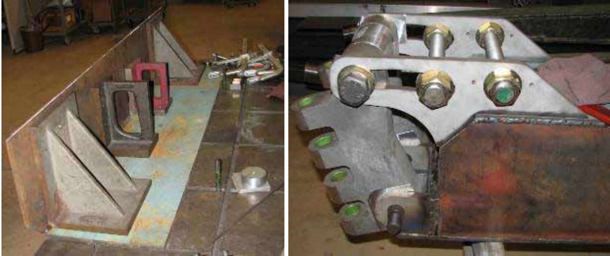
Figure 4.19: Left: 1 st step complete clamps have been removed. Right: 7 th step, critical placement of the Lower Adjustment Brackets. Hinges, all thread, and shims are used to jig into place. Consider tack welding on some straps across the brackets to further constrain warping.
