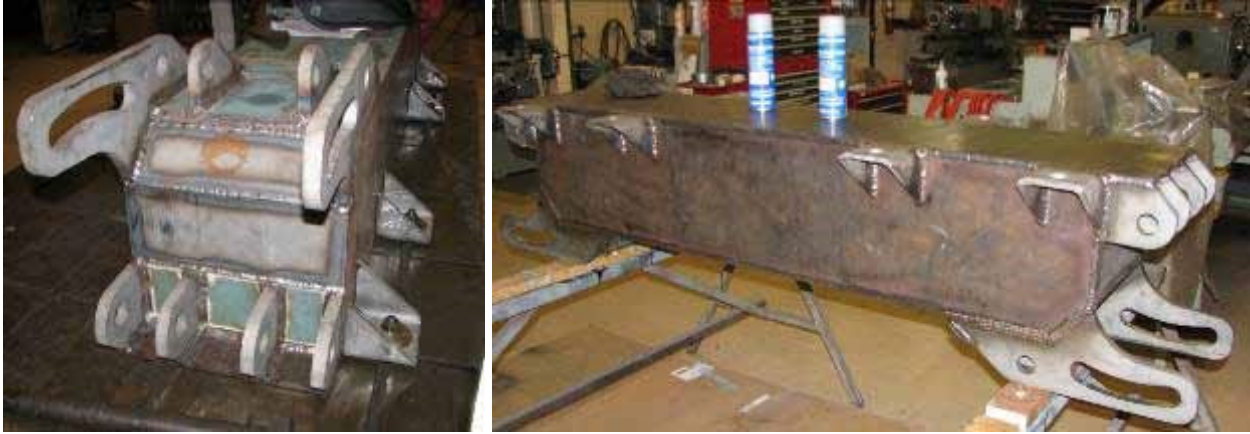
Figure 4.21: Left: 13 were touched up and cleaned to be painted. th step attachment of Mounting Brackets. Right: final Inboard Beam fabrication; the welds
