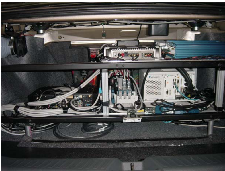
Figure 20. Trunk rack system
