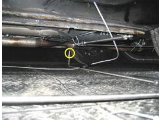
Figure I-9. Hydrogen leak straight up from tank position underneath automobile.
